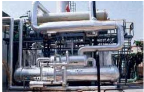
Figure 8: Transparent Energy Systems PVT Ltd absorption refrigeration system (TES PVT Ltd, 2007).
